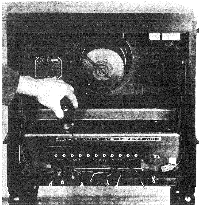
Figure 6—Removal of R.P.A. connections, Radiotrons and Rectrons preparatory running continuity tests
